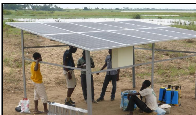
Pilot Project: 2.5 kWp field irrigation system using VFD and a surface water pump (Aveyime, Volta)
