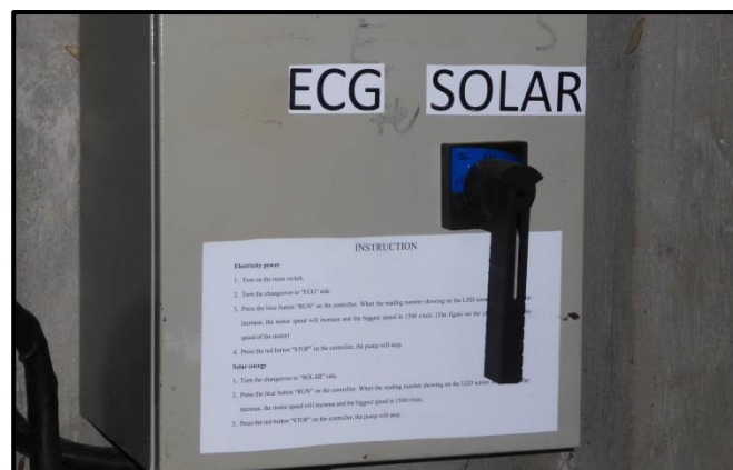
Change-over-Switch between PV Solar and ECG (Electricity Company Ghana) to run a 37kW irrigation pump via VFD control (Aveyime, Volta)
