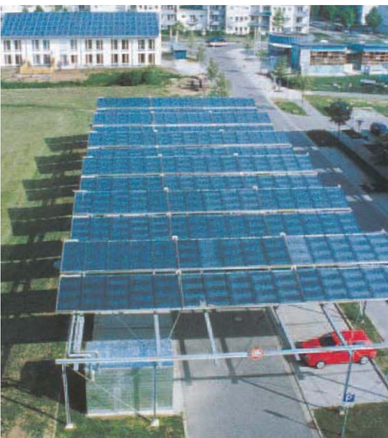
In Neckarsulm even the parking spaces are used for generating heat.
