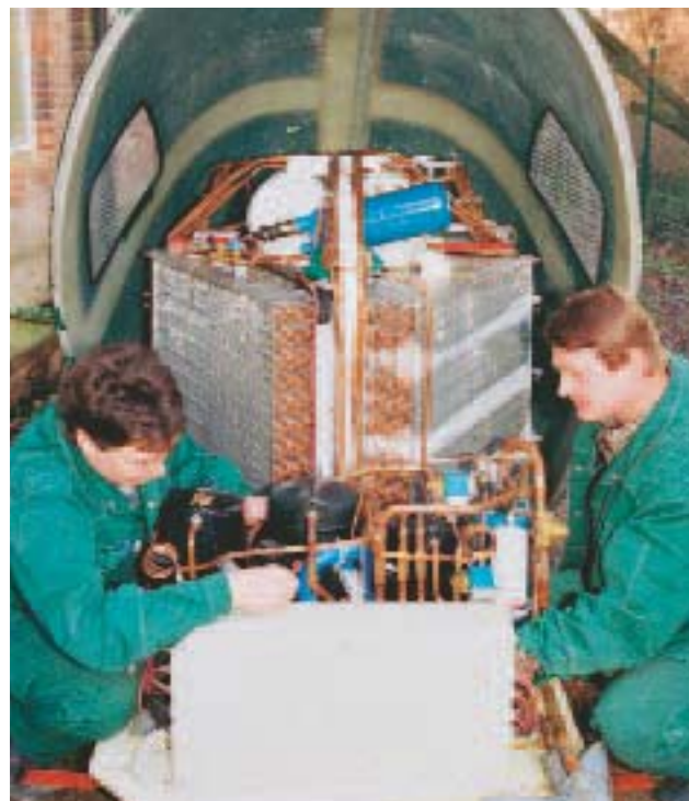
Maintenance work on a heat pump which uses ambient air for heat production
