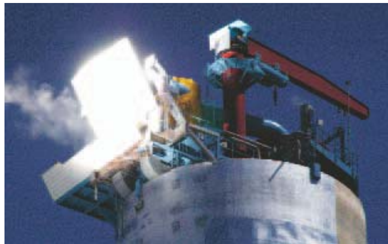
Receiver and engineering systems in operation at the top of the tower
