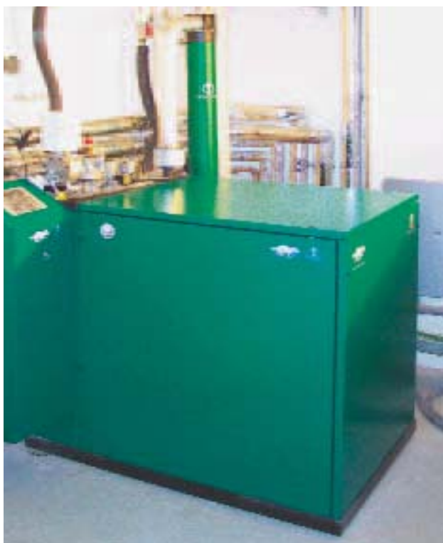
Motor cogeneration plants come in different sizes: large (above) and small (below).
