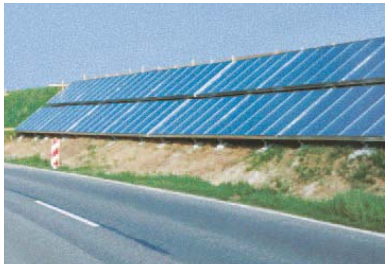
Solar collectors both heat residential areas and protect them from noise.
