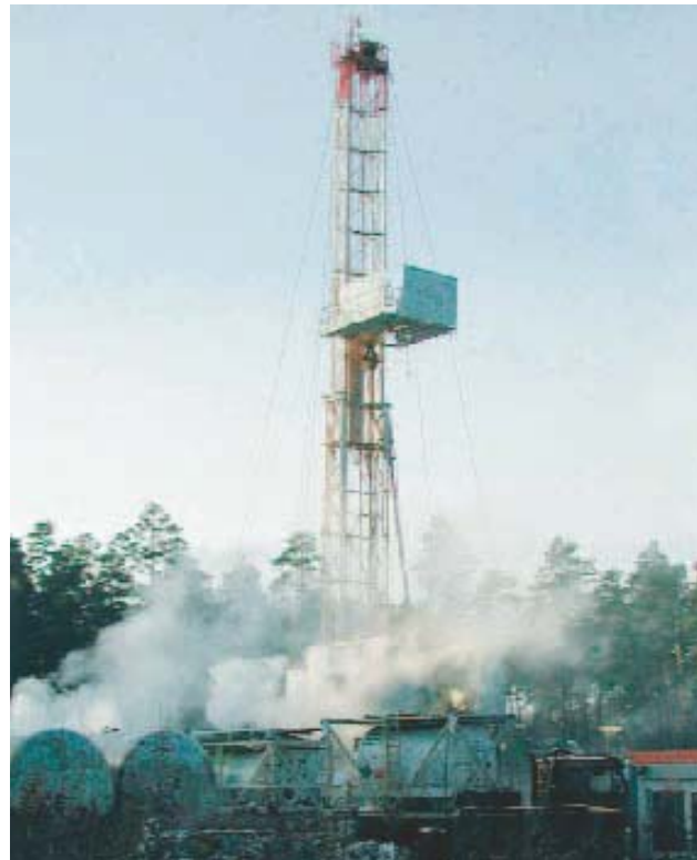
Geothermal bore hole in Groß Schönebeck
