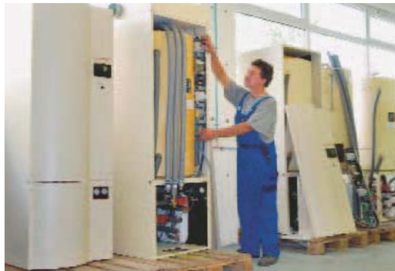
Some series of heat pumps are designed to fit easily in the interior decoration of a house, e.g. in a kitchenette
