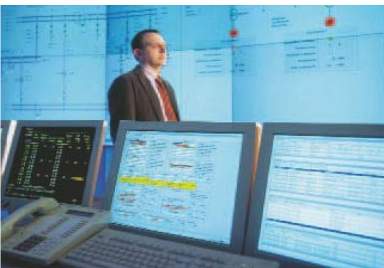
In this control room belonging to the STEAG Saar Energie, power plants and disengageable consumers are linked nationwide. The STEAG markets this power for grid regulation.
