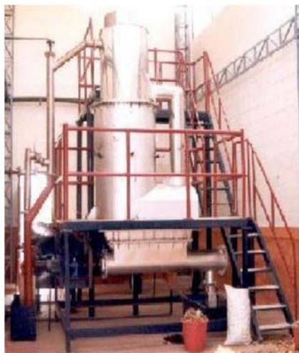
Figure 3.4: View of 75 kW gasifier at CART
